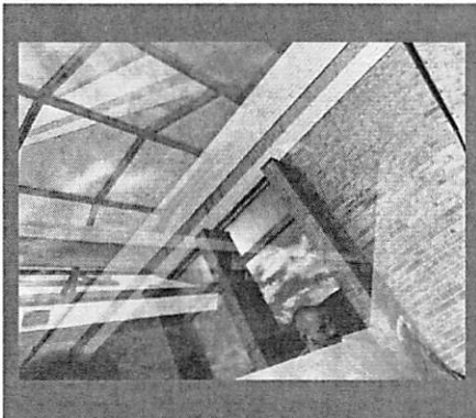
Typical interior condition showing water damage
