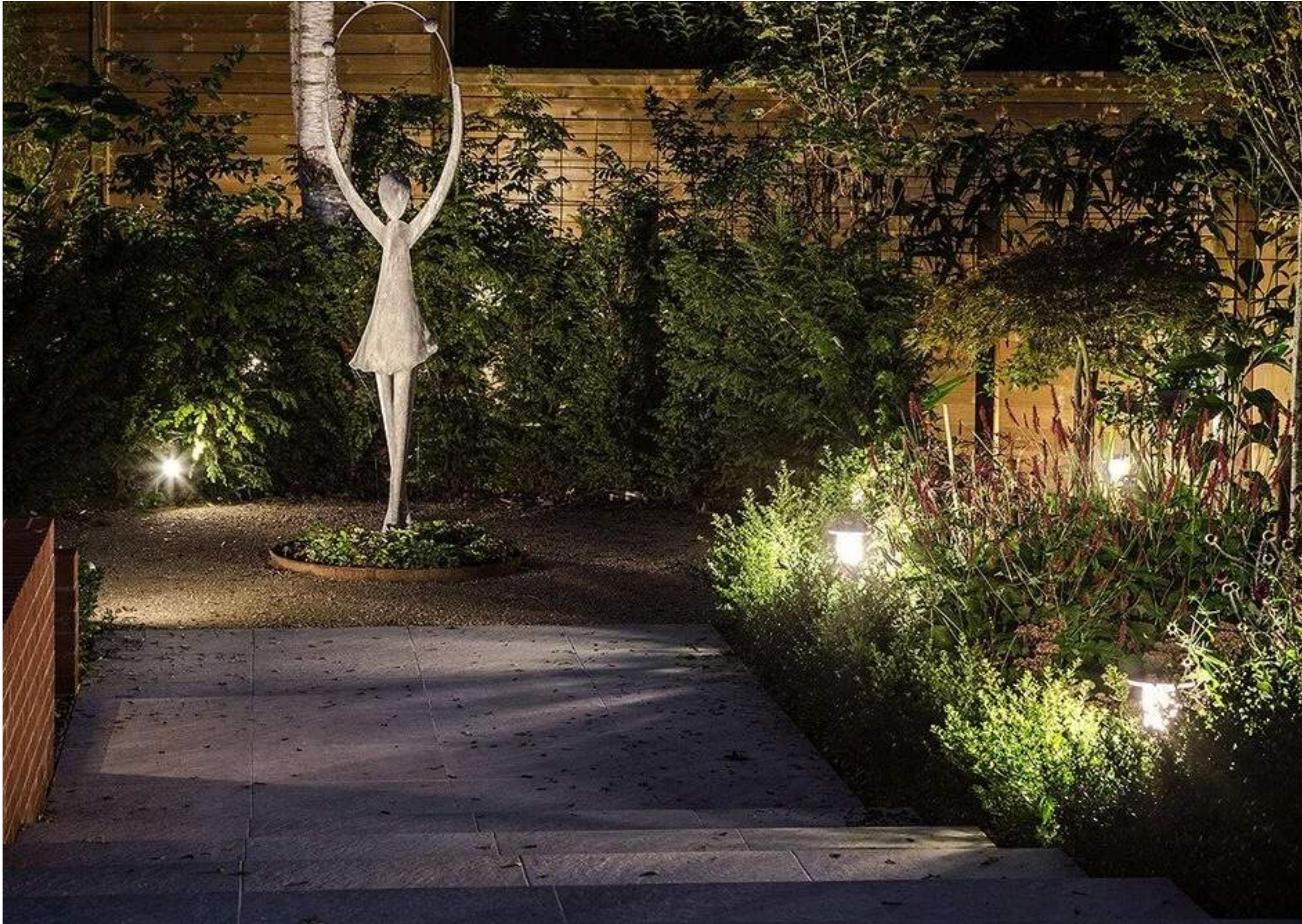
PATHWAY LIGHTING (LOW VOLTAGE)
