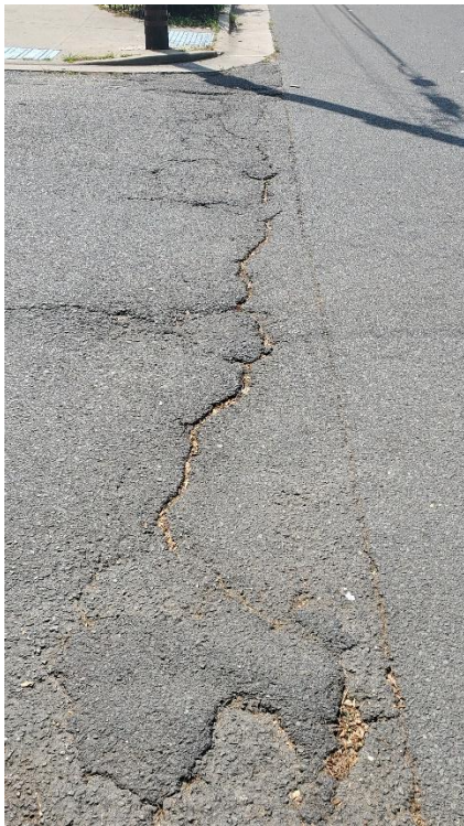
Longitudinal Cracking and Vegetation Growing in Roadway
