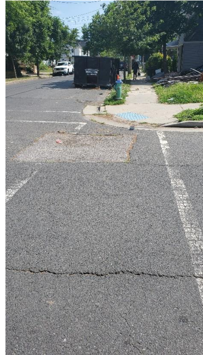
Non-Compliant Handicap Ramp, Centerline Cracking, Roadway Patches, Faded Traffic Marking Lines
