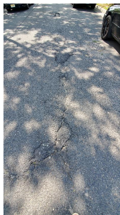
Centerline Cracking, Roadway Cracking, Roadway Patches
