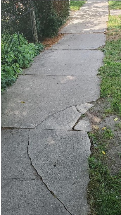
Non-Compliant ADA Accessible Route and Cracked Sidewalk
