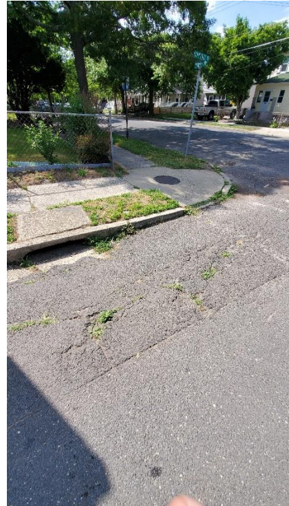
Non-Compliant Handicap Ramp and Non-Compliant Type B Inlet
