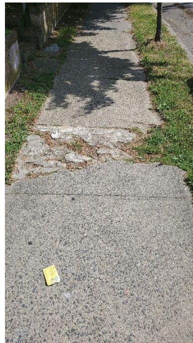
Non-Compliant ADA Accessible Route, Cracked Sidewalk
