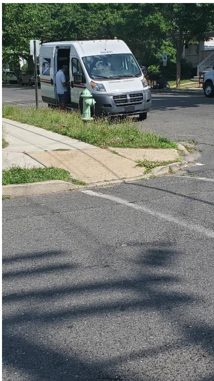
Non-Compliant Handicap Ramp
