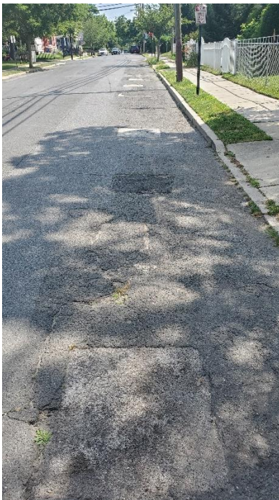
Roadway Patches, Alligator Cracking, Vegetation in Roadway
