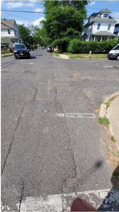
Roadway Trenching, Non-Compliant Handicap Ramp, Faded Traffic Marking Lines
