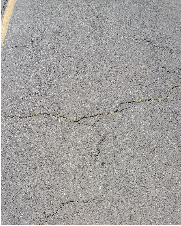
Transverse Cracking and Vegetation Growing in Roadway
