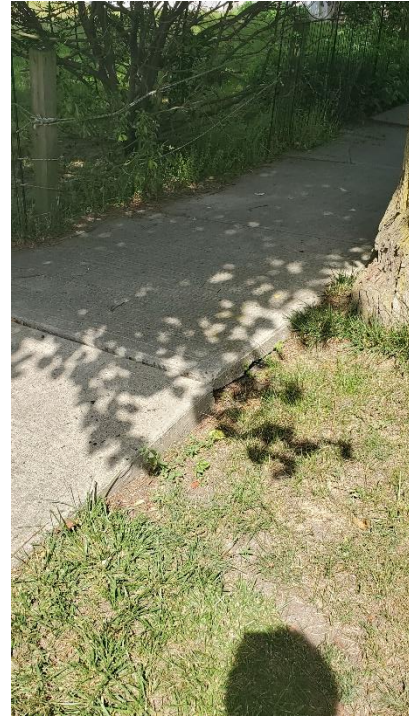
Non-Compliant ADA Accessible Route, Heaved Sidewalk
