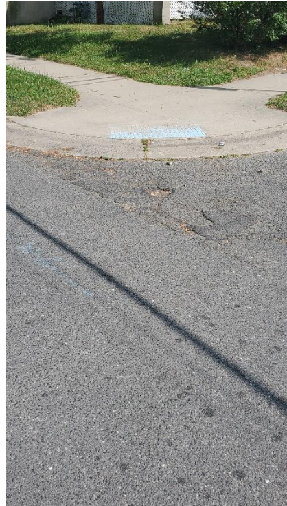
Non-Compliant Handicap Ramp and Potholes
