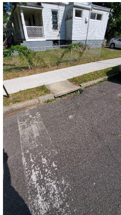
Non-Compliant Type B Inlet and Faded Traffic Marking Lines
