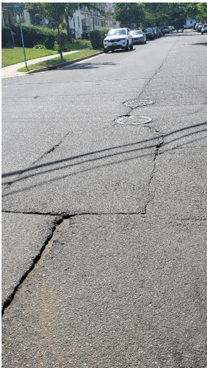
Centerline Cracking, Roadway Cracking, Roadway Patches
