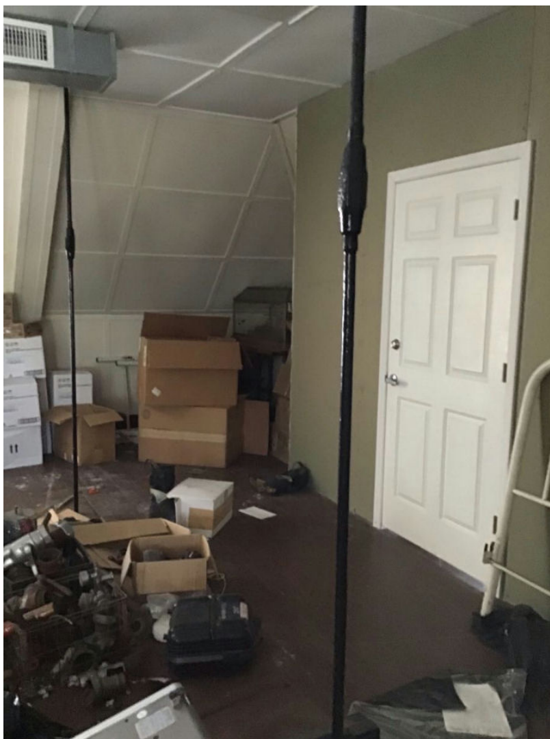
11 11-Pre-Mitigation - Document Date Taken: 7/16/2021 Room (Zone 1) 8
