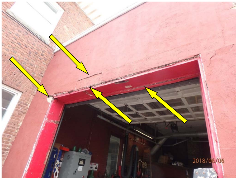
Bay door #1 with cracked/displaced plaster finish and deteriorated timber door framing.
