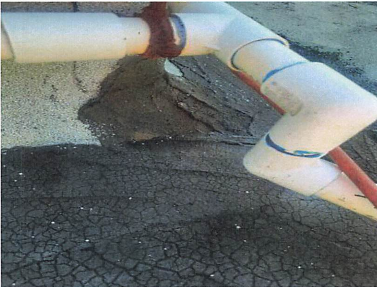
leaking at rtu
