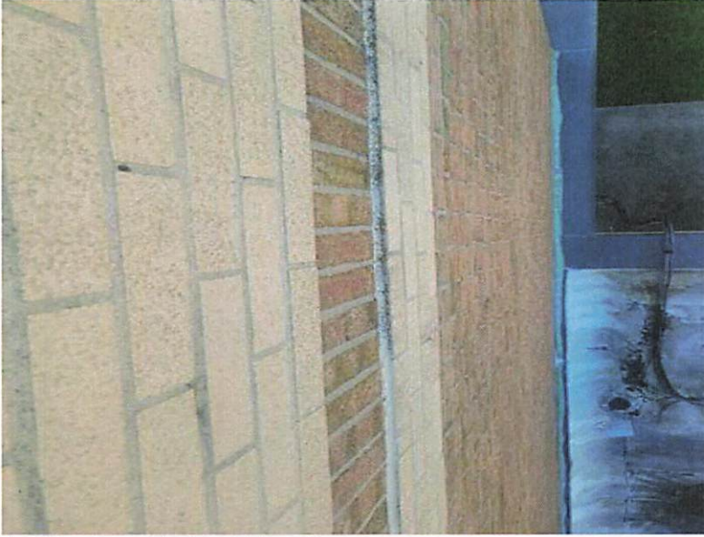
deteriorating sealant outside wall
