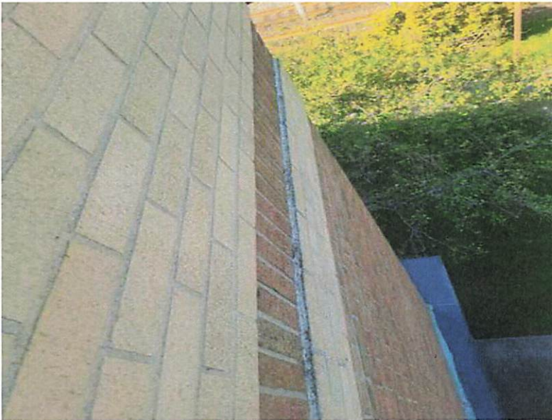
deteriorating sealant North West outside corner
